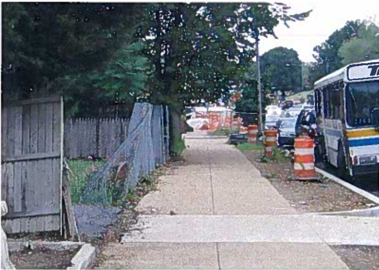
1414 Maryland Avenue – Illegal fence protrudes into sidewalk endangering pedestrians
