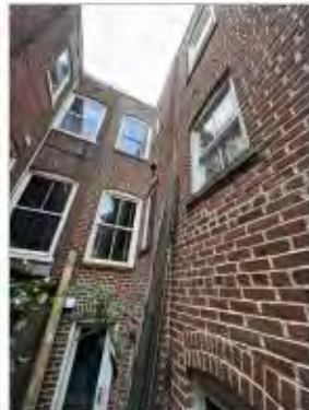
VIEW OF DOGLEG CONDITION FROM GROUND LEVEL
