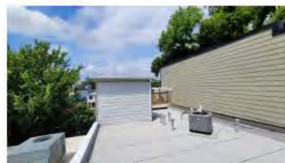
VIEW 7 FROM FRONT PORTION OF ROOF TOWARDS EXISTING ROOF DECK AND NEIGHBOR'S PARTY WALL
