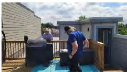
VIEW 6 EXISTING ROOF DECK LOOKING TOWARDS STAIR POP UP AND TOWARDS FRONT OF HOUSE IN DISTANCE
