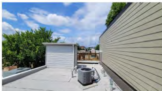
VIEW 8 FROM FRONT PORTION OF ROOF TOWARDS EXISTING ROOF DECK AND NEIGHBOR'S PARTY WALL
