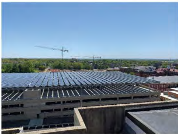
Children's National Research Center Parking Lot, 1.1 MW
